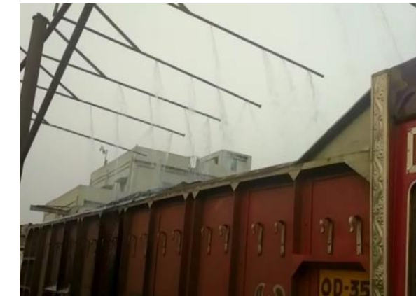
WAGON SPRINKLING SYSTEM
